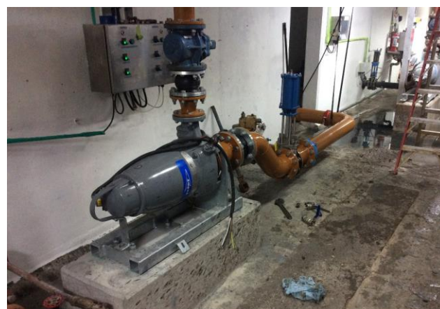
Figure 6 – Replacement sludge pump, Guarding not required
