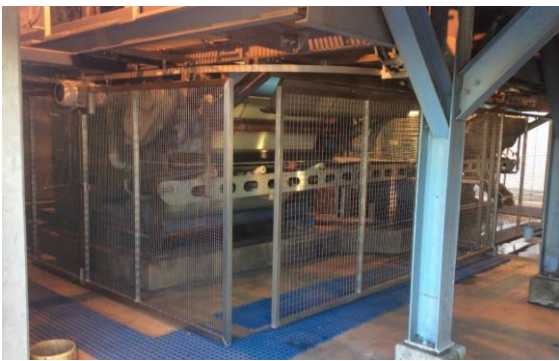
Figure 4 – Guarded belt press (partial install)
