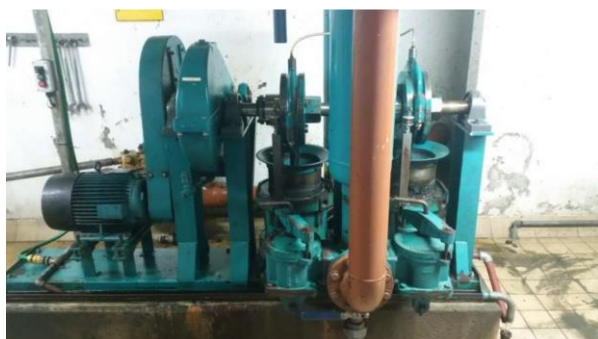
Figure 5 – Existing sludge pump, requiring guarding
