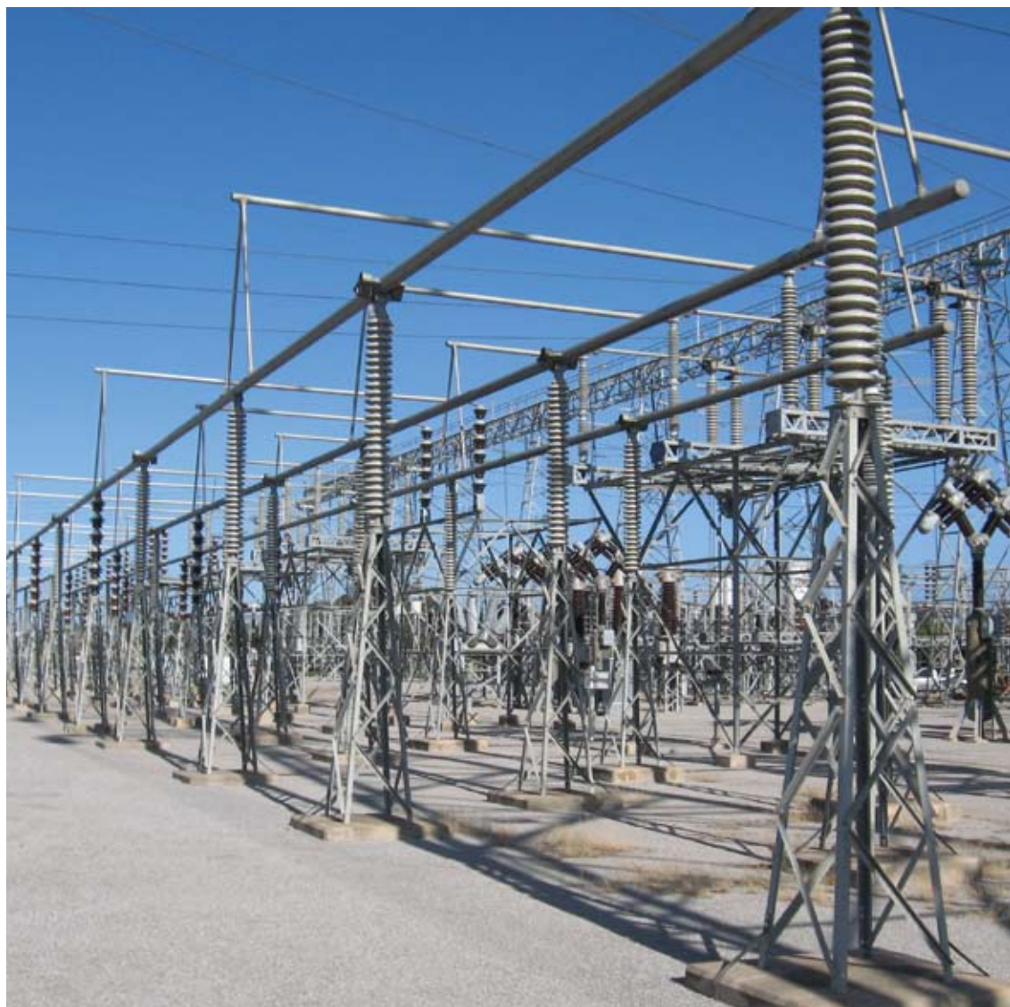
Geelong Terminal Station (see story inside)
