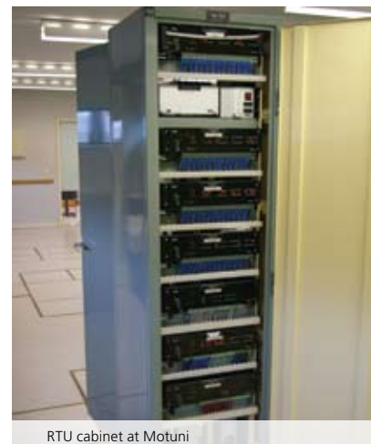
RTU cabinet at Motuni
